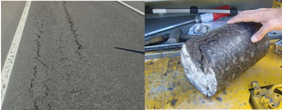
Figure 1-1 Pictures showing the development of top-down cracking
