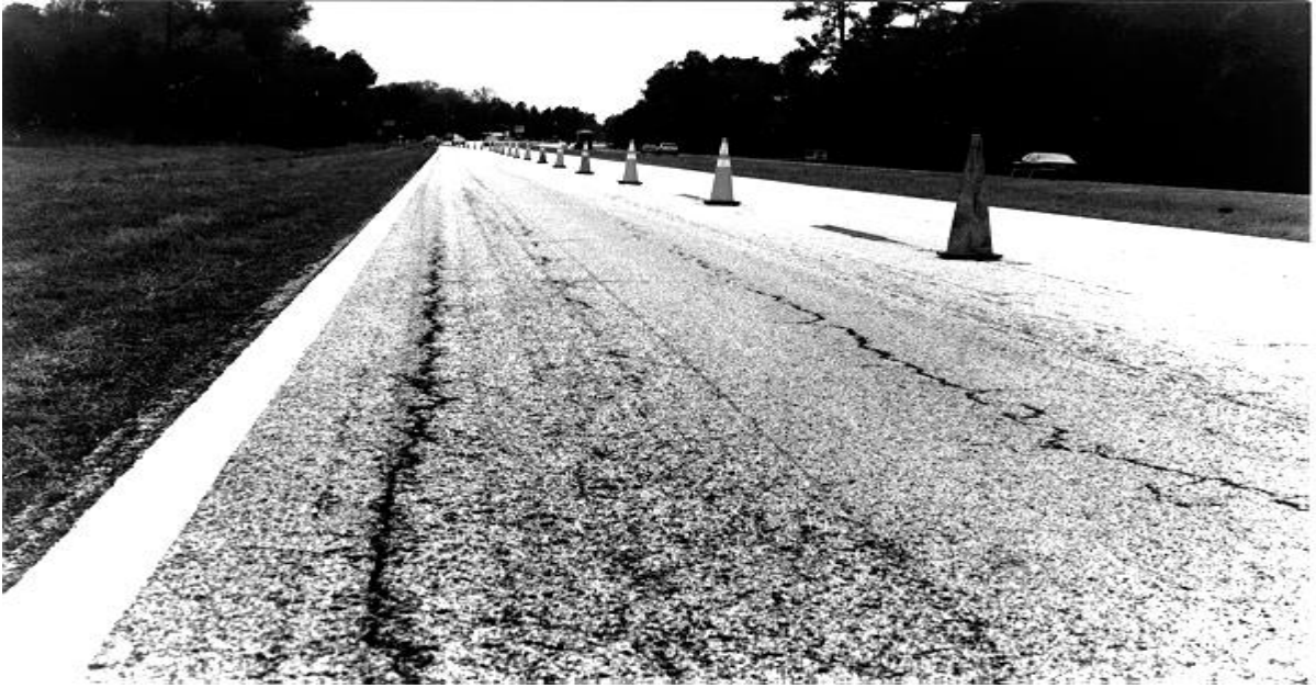
Figure 2-10 Lane exhibiting surface initiated top-down cracking in both wheelpaths (Myers et al., 2000)
