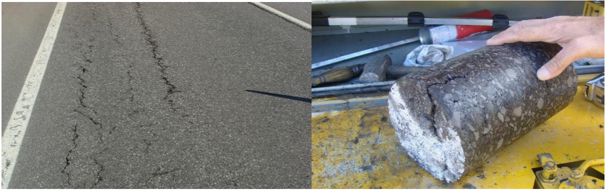
Figure 6-1 Photos showing the development of top-down cracking
